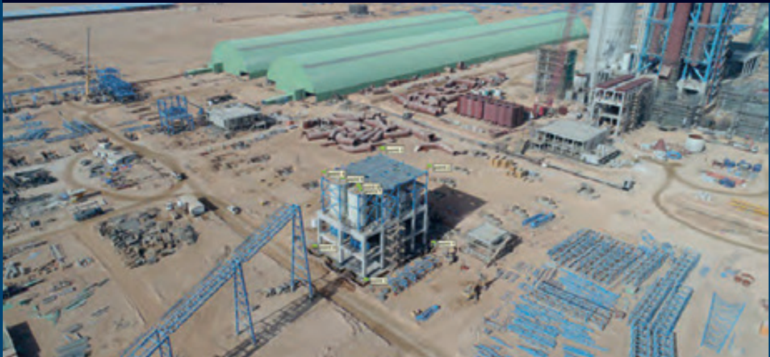
Concrete Plant, Saudi Arabia
